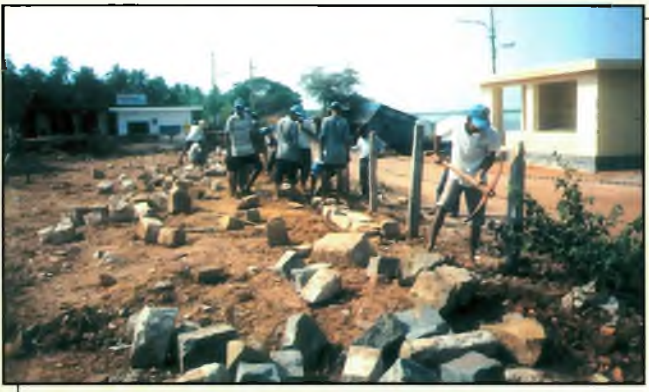
NSS Volunteers leveling the play ground at ZP Higher Primary School, Balekudru
