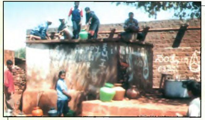
NSS Volunteers participating in the cleaning operation of water tank as a part of Shramadana in NSS Camp held at Hanumanthawadi (B) village
